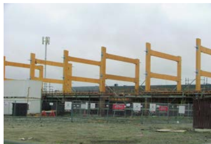
Trimble (Christchurch) 2 storey post tension office block. LVL fabricated columns, floor and roof beams
